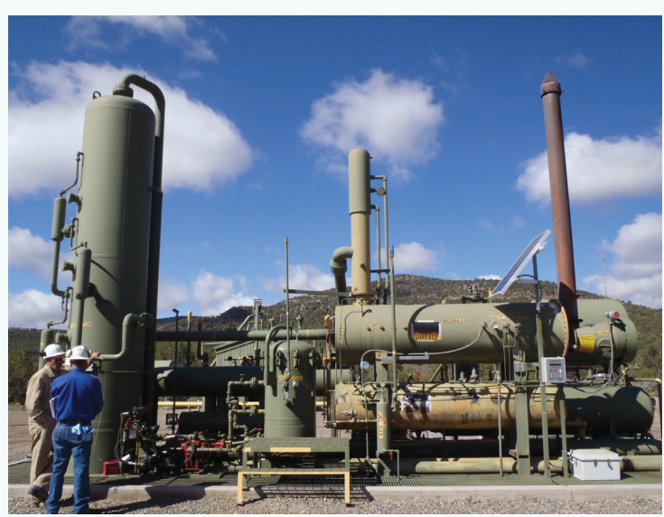
A glycol dehydration unit at a natural gas compressor station: one of many synthetic minor sources of air pollution on the Southern Ute Indian Reservation.
