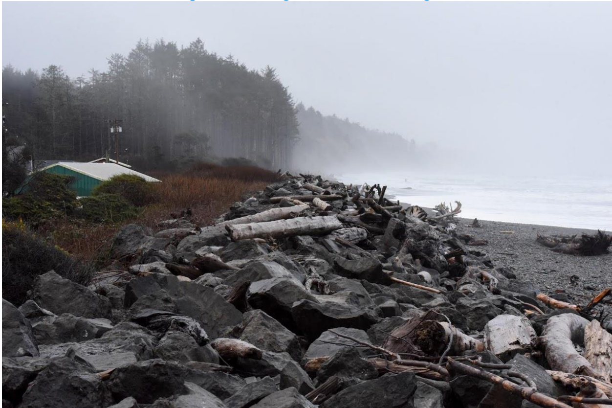
A seawall, damaged by storm surges and high tides, stands along the coastline near Quinault Indian Nation's main village. REUTERS/STEPHANIE KEITH
